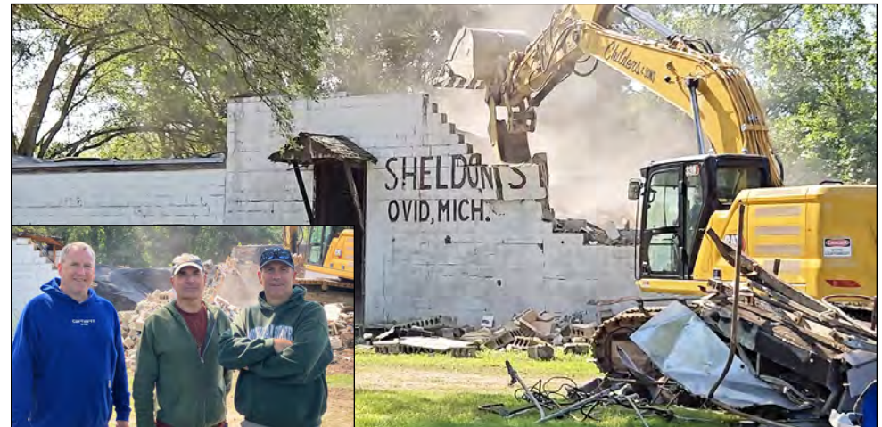
Sheldon Packing House being raised on Monday, August 12, 2024. Insert: Brothers Scott, Greg and Allen Martin watched the demolition. Photo by Allen Martin
